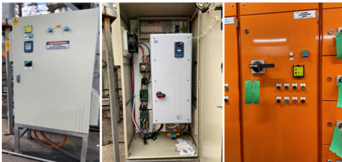
Figure 13 VSD Panel of a new blower and power supply from WestVAMP Plant.
